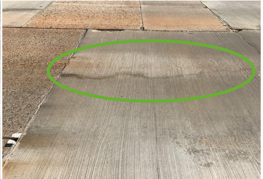
Control – Visible Crack Across Slab
