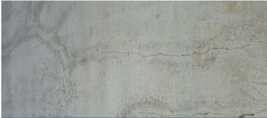
Control Trial Slab after 6 months Significant cracks and evidence of wear
