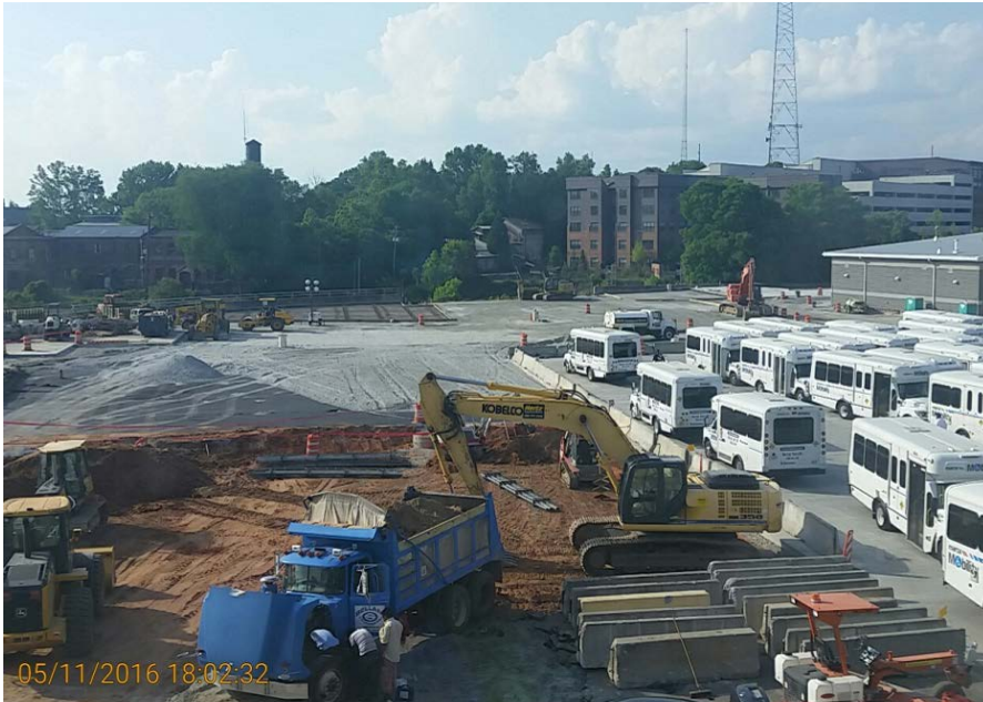
MARTA Brady Mobility Facility – Trial Concrete Slab Heavy Duty Wear/ High Abrasion Application
