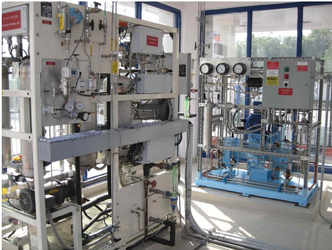
Figure 2 The electrolyser and compressor at the Dwarka Hythane® Station
