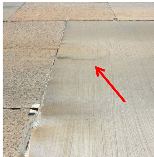
Figure 4. Control - Visible Crack Developing
